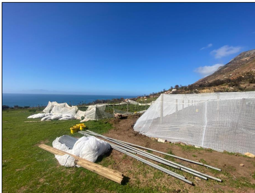
Figure 6. The vegetable tunnels at Rocklands Farm are currently under repair.
